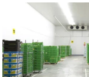
Cold Storage & Freezer Rooms
