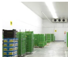
Cold Storage & Freezer Rooms
