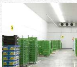
Cold Storage & Freezer Rooms
